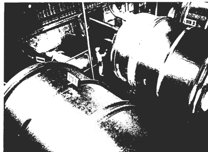
Fig. 6. View of converters and compressor. (Photo courtesy of U.S. Energy Research and Development Administration)
